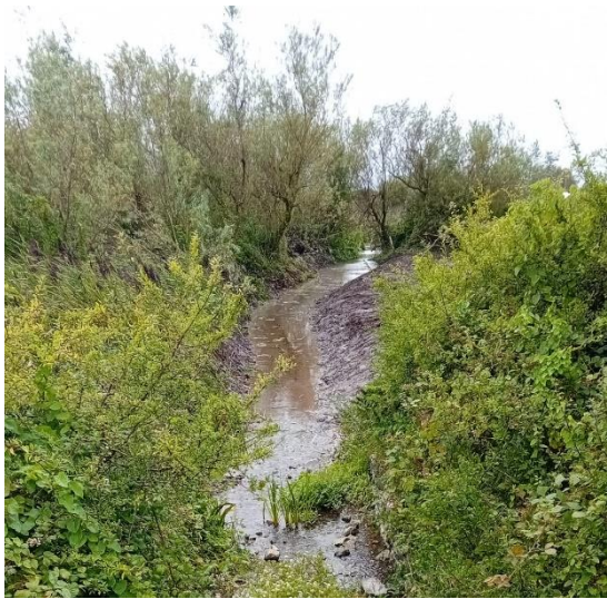
KILLEENARAN, REMOVAL OF IN-STREAM VEGETATION BLOCKAGE
