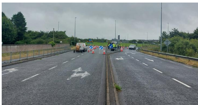
PEDESTRIAN BARRIER REPAIR WORKS ON THE R446/N65 INCLUDING EXTENSIVE TEMPORARY TRAFFIC MANAGEMENT AT LOUGHREA
