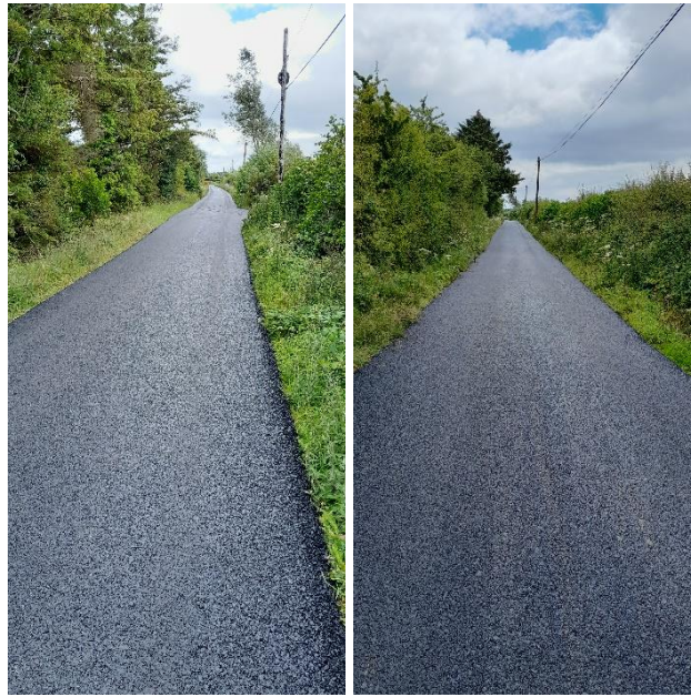
(RI) RESTORATION IMPROVEMENT, AT CURRAGHLENAHANAGH - DBM WORKS IN ADVANCE OF SURFACE DRESSING
