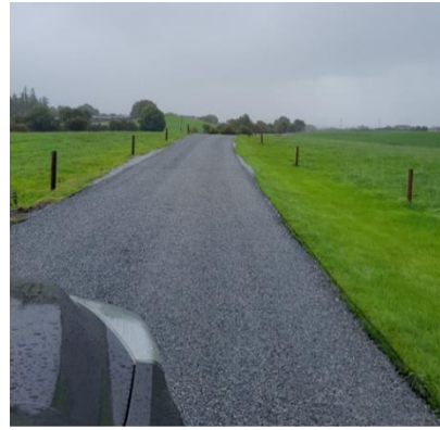
BEFORE AND AFTER IMAGES OF A PRIVATE ROAD FOLLOWING WORKS CARRIED OUT UNDER THE LOCAL IMPROVEMENT SCHEME WORKS, DUNIRY
