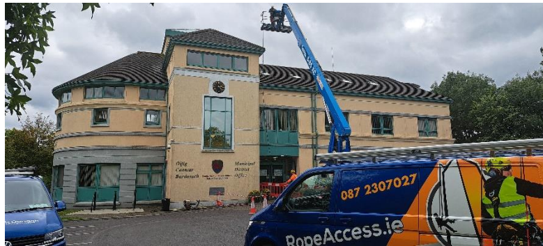
BALLINASLOE MD OFFICE ROOF INSPECTION & REPAIRS COMPLETED IN CONJUNCTION WITH GALWAY COUNTY COUNCIL FACILITIES SECTION
