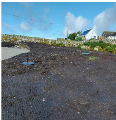
BEFORE AND AFTER PHOTOS SHOWING THE OLDER INSTALLED TREATMENT PLANT ON THE LEFT WITH THE NEW TREATMENT SYSTEM ON THE RIGHT
